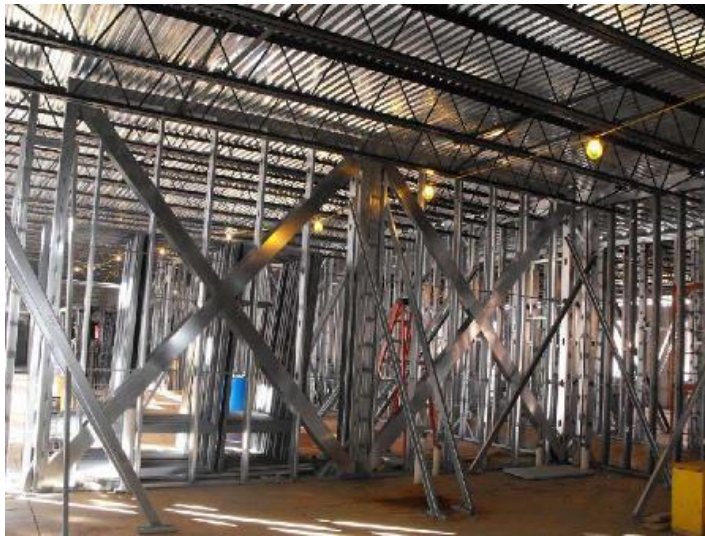
Shear resistance was provided by CFS strapping welded to both bearing panels and partitions. Strap-braced walls were shop-fabricated and bolted in place. Photo by DSi Structures
