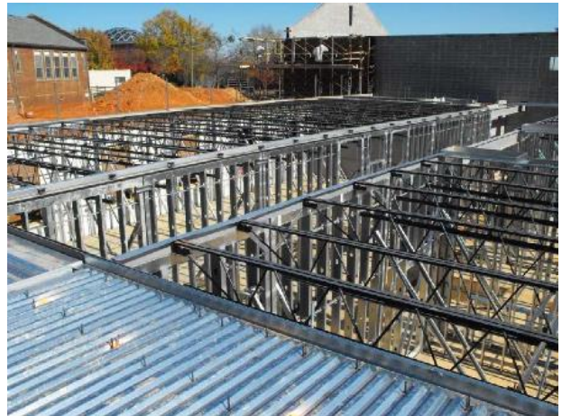
Loadbearing panelized CFS walls in front of existing brick structure under renovation. Load distribution members negated the need for alignment framing. Composite headers reduced framing above the openings. Photo by DSi Structures
